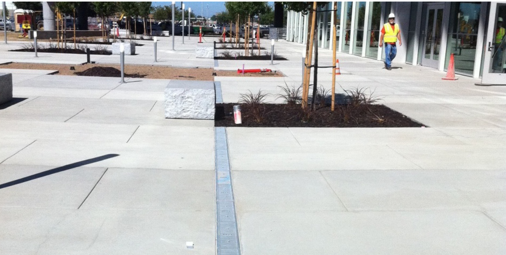
Above Right: Detail of Installed Dura Slope with Cast-Iron Grate Above: The Finished Installation
